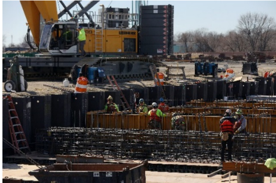
Workers construct a wharf at the Paulsboro Marine Terminal. The port, built on the site of a former oil terminal, will soon be home to a manufacturing facility for the German company EEW to build monopiles for offshore wind turbines. TIM TAI / Staff Photographer
